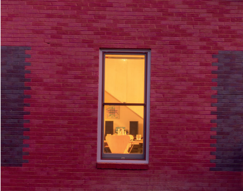
2023 Detail of Third Street Elevation. Color wraps the corners and marks the locations of original bay geometry and windows discovered during interior demolition. Photo by Robert Batey Photography.
