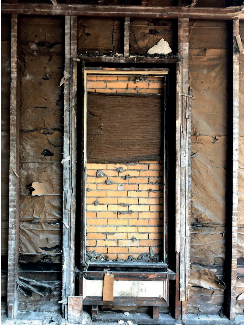
SEPT 2020 Recovering material to repair and replace or reposition during demolition and deconstruction.
