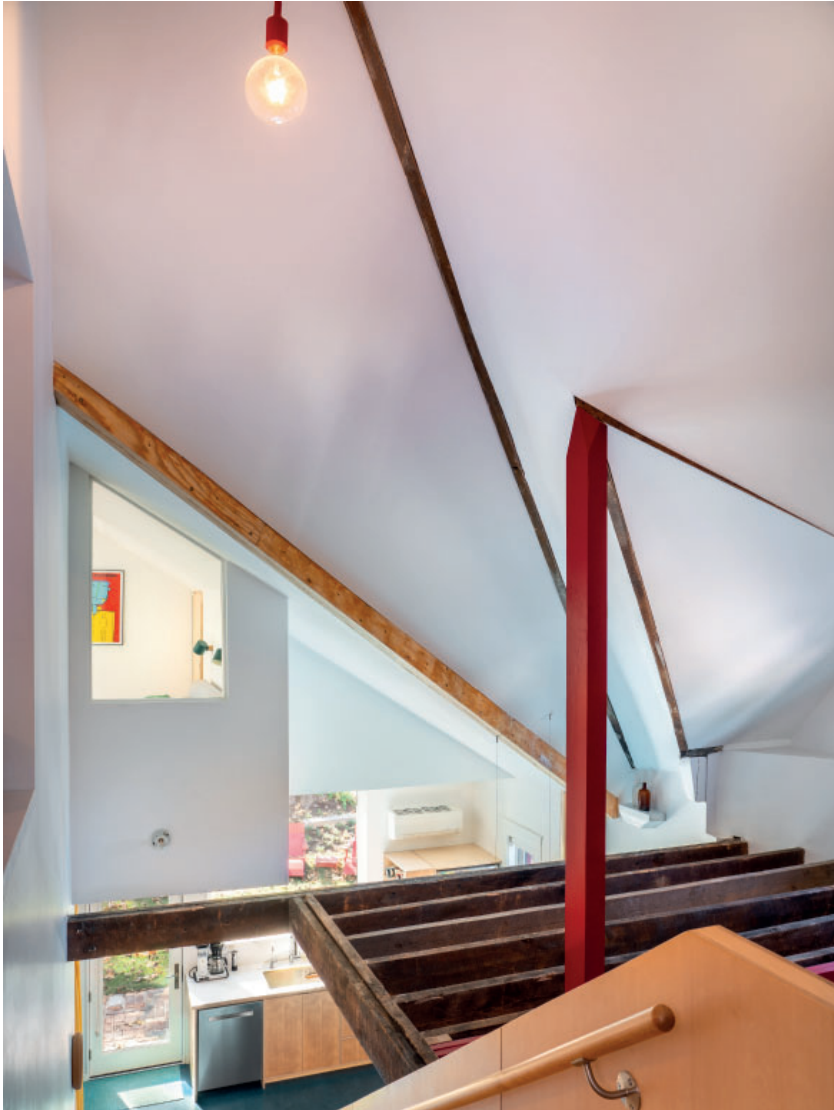
2023 Interior Upper Level. New (red) posts and salvaged (white) blocks provided needed support for an existing dormer. Existing ceiling joists were uncovered, cut in place and doubled/headered to create a stair void. Photo by Robert Batey Photography.
