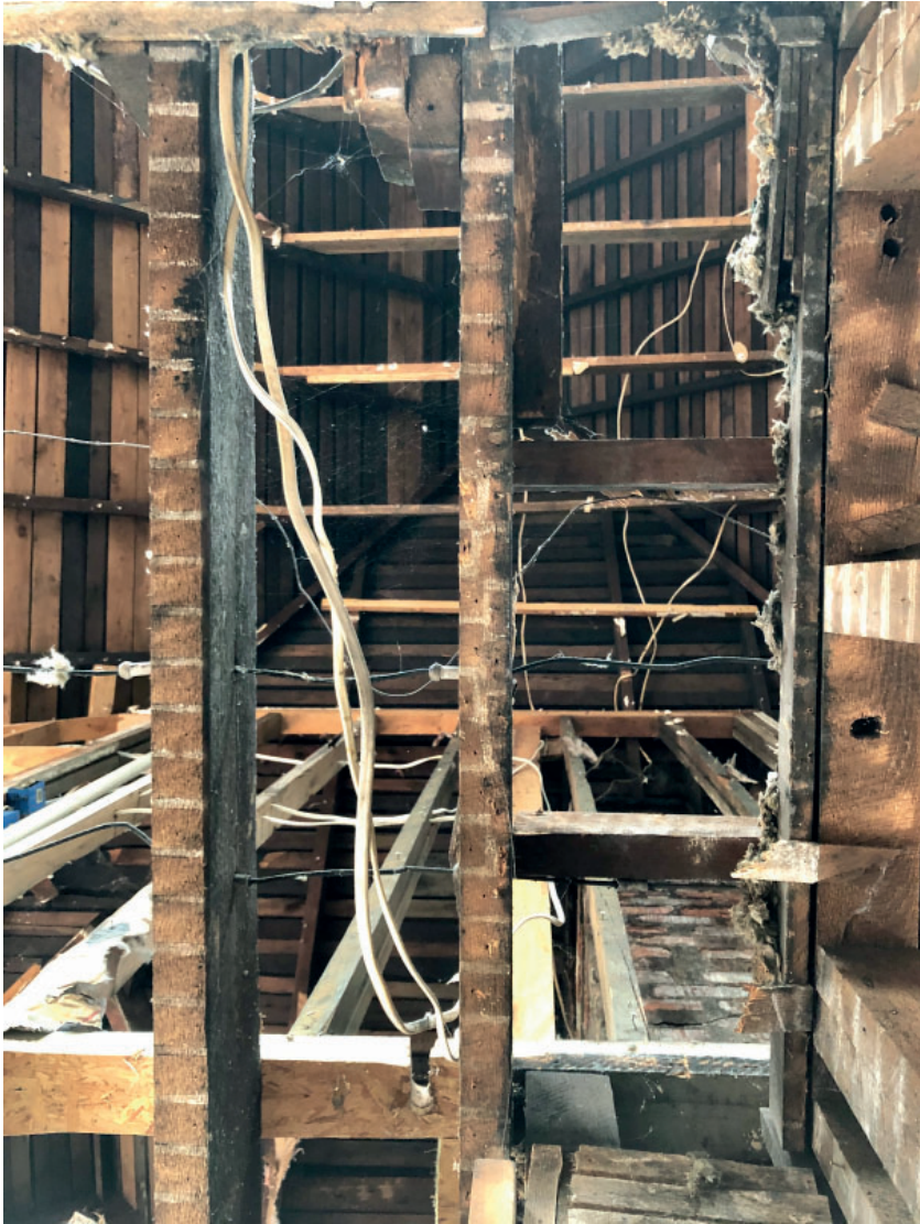
SEPT 2020 View through joists with exposed lath marks to attic wall and roof framing and skip sheathing.
