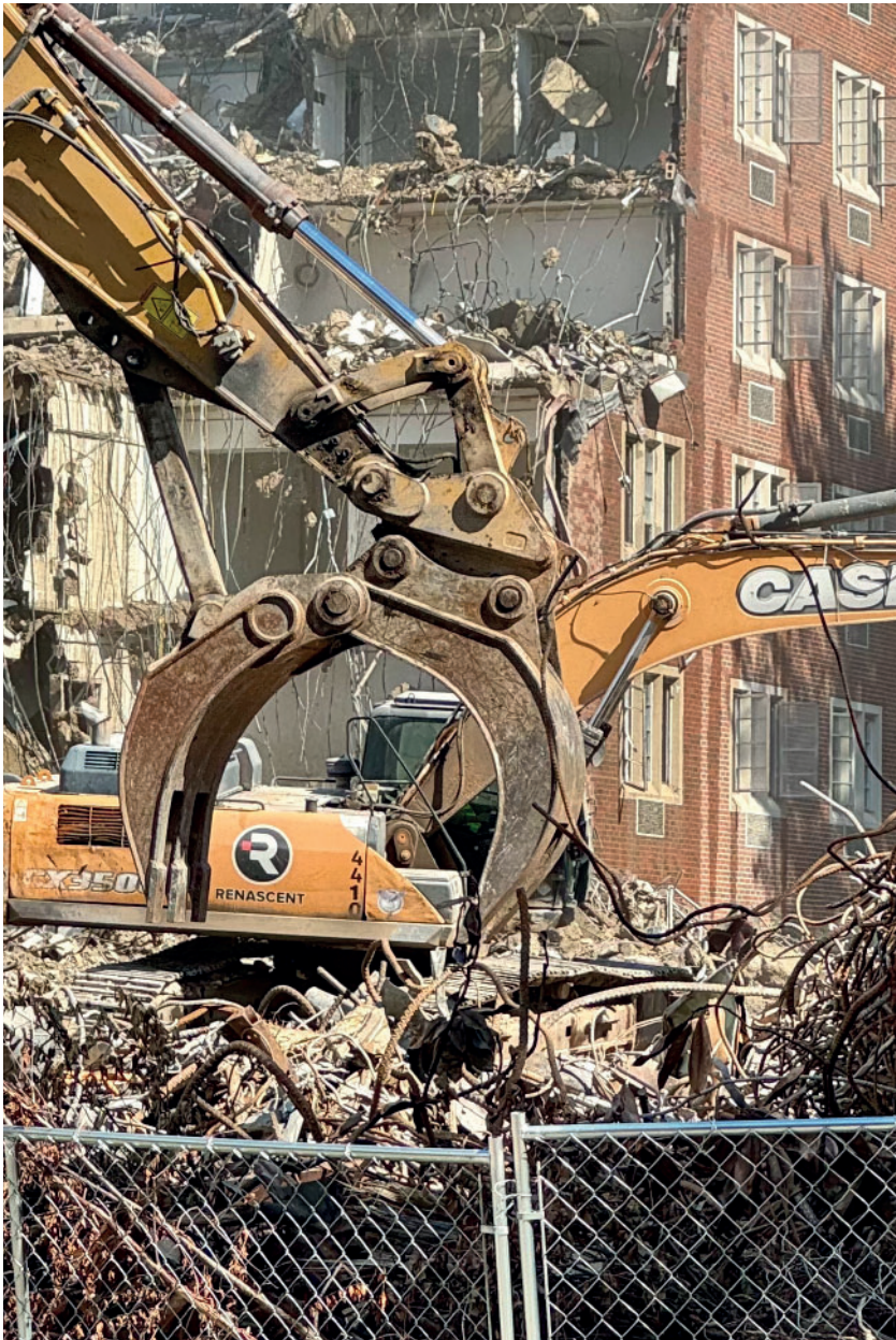
MAY 2024 Demolition of four residential halls and one classroom building to make room on this site for a new classroom building despite the university's stated immediate need for 1.4 million gross square feet of housing (Per Chancellor's address and University Master Plan Slide Presentation . Photo by Author.
