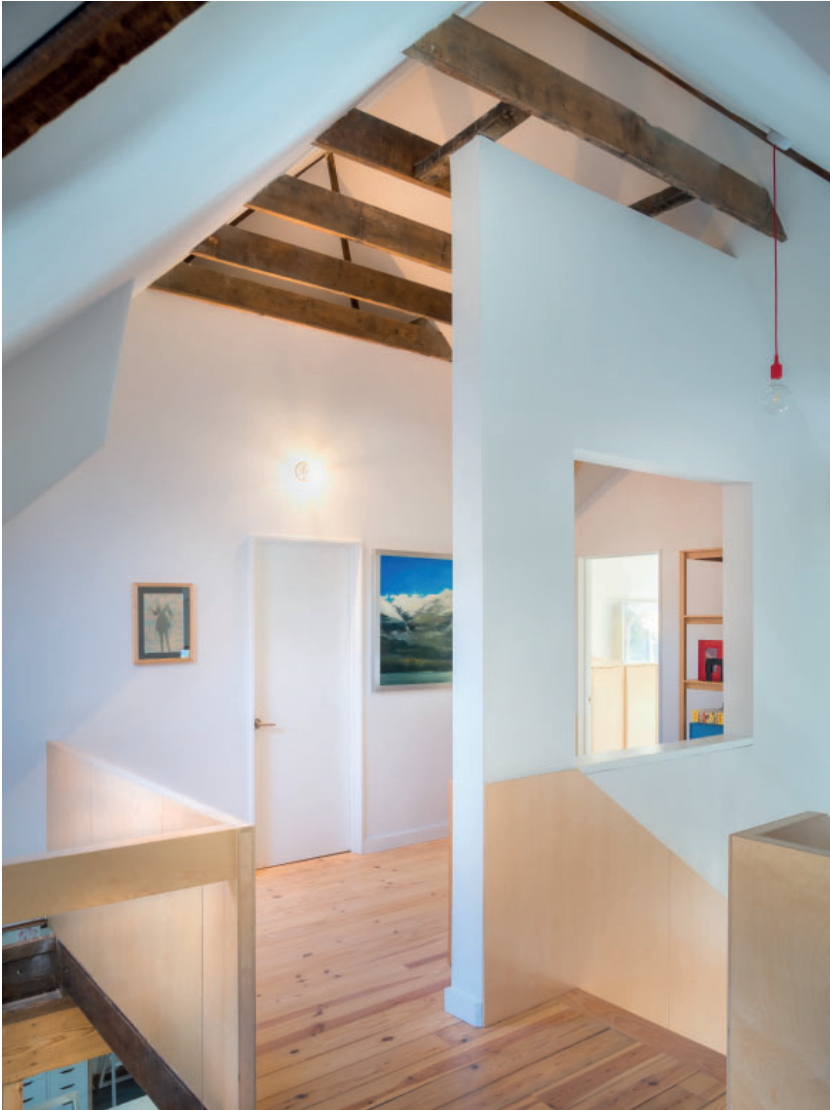
2023 Interior Upper Level. Existing framing was leveled and voids created. Collar ties were exposed, retained, and lightly cleaned. Structure heart pine decking was salvaged from downstairs, de-nailed, planed, and reinstalled adjacent to new structural pine decking. Photo by Robert Batey Photography.
