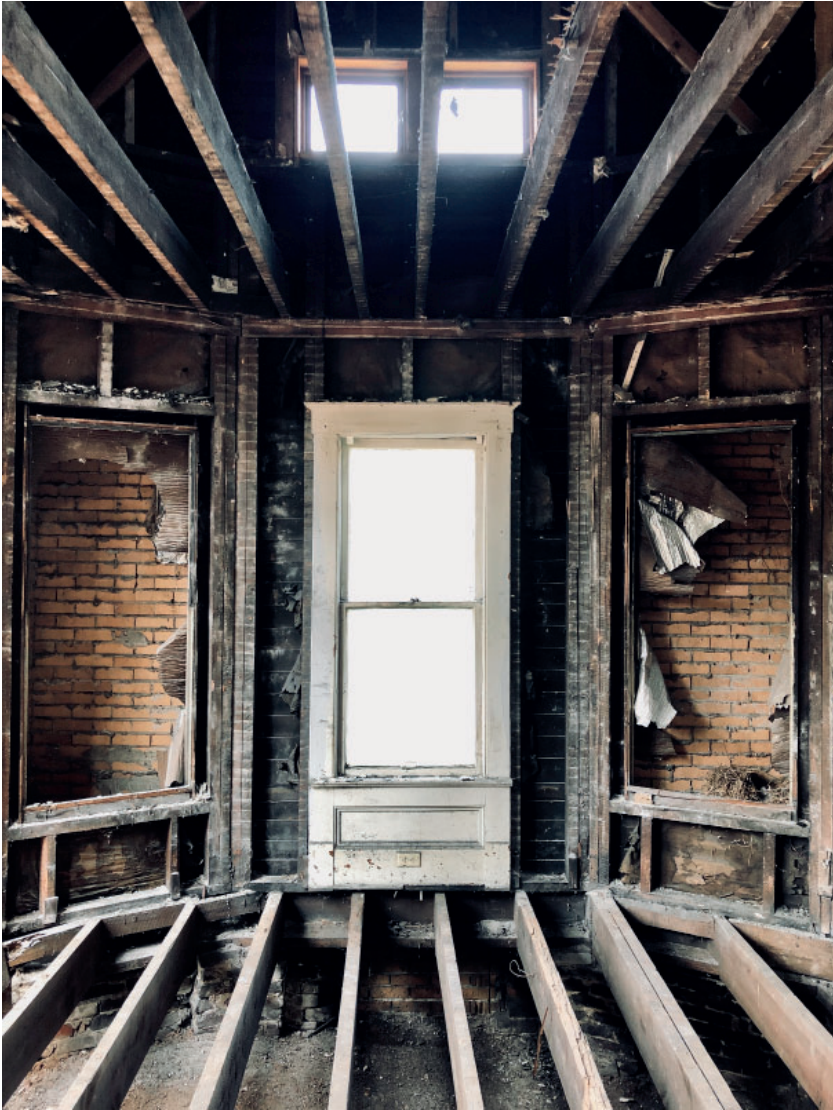
SEPT 2020 Removal of finishes presented voids between original bay windows and outer brick shell.
