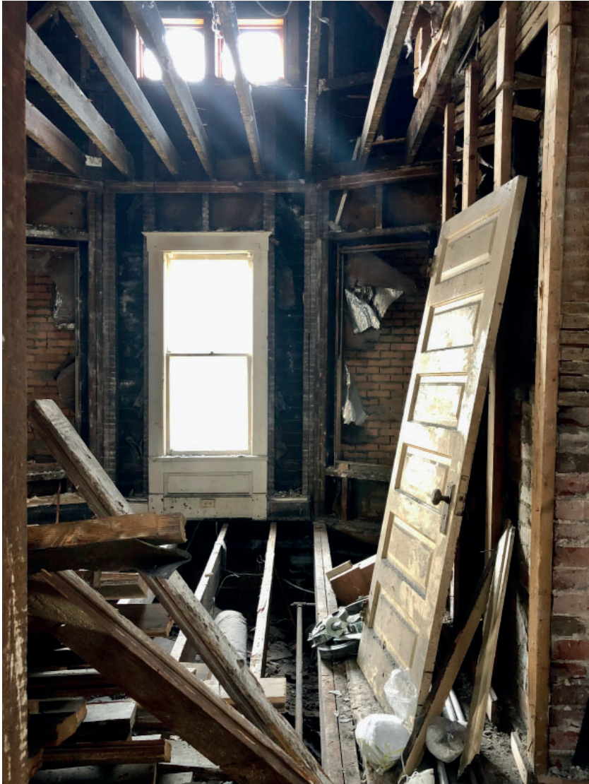
SEPT 2020 Recovering material to repair and replace or reposition during demolition and deconstruction.
